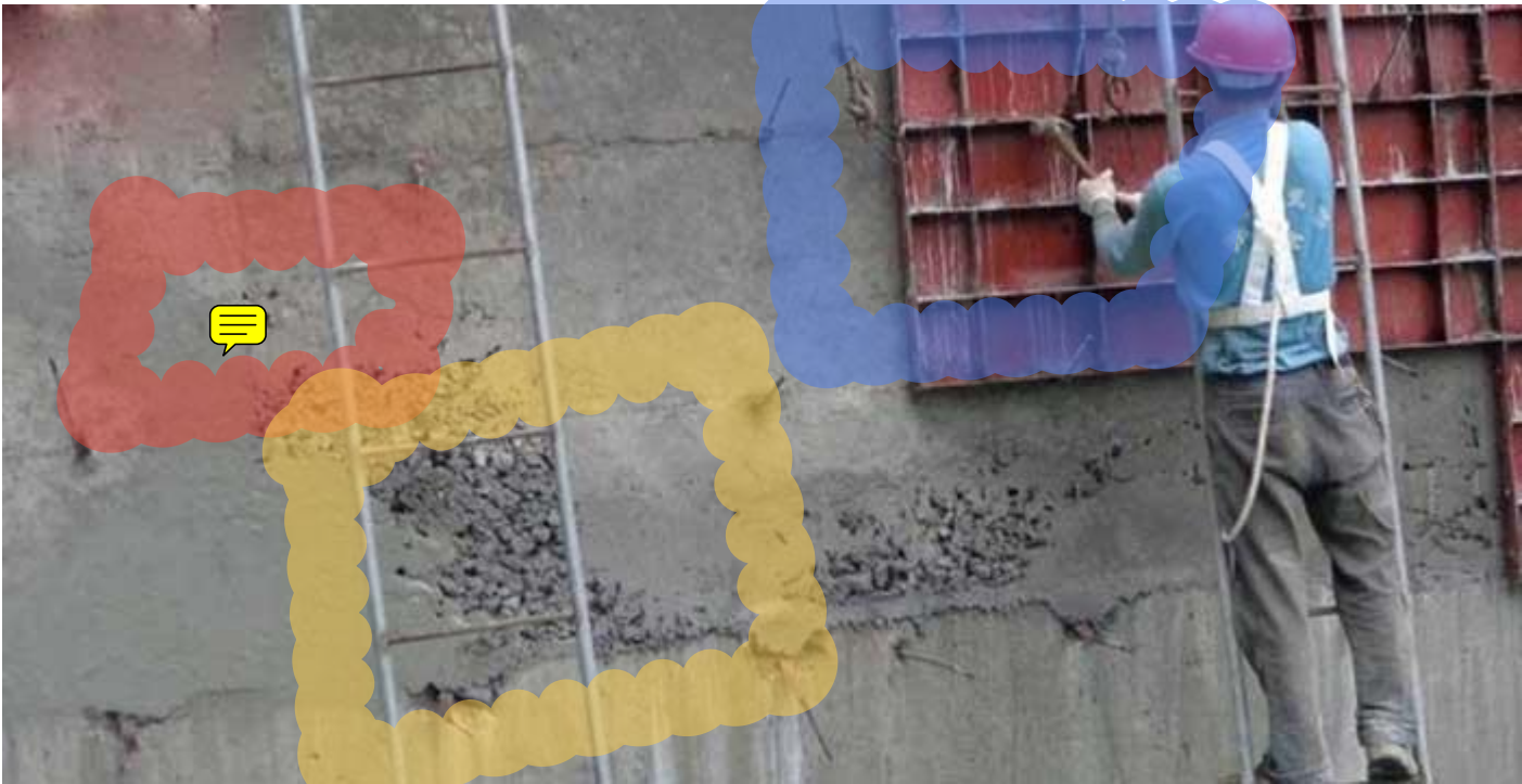
Sample 2: Opacity 50% & Stroke 20pt: Concrete defect
